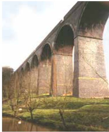
2 One of four impressive viaducts within this character area built in 1902, carrying the South Wales to London railway over the River Frome valley. Taken from the Frome Valley Walkway.
